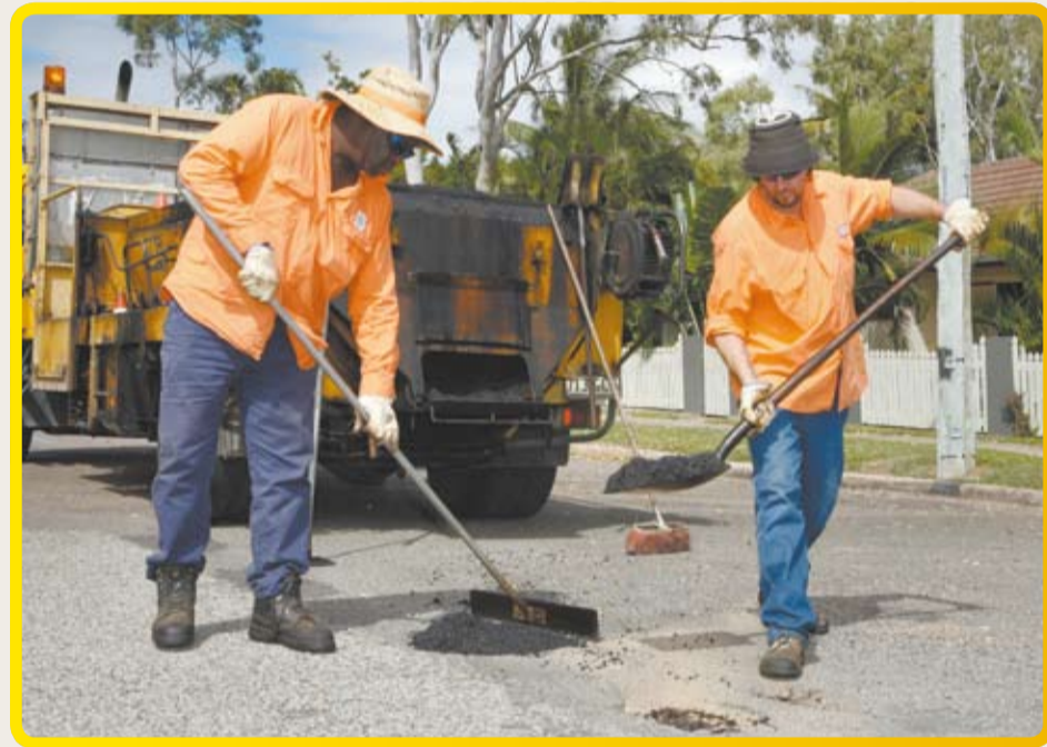
Crews are busy filling potholes in the wake of the wet season.
