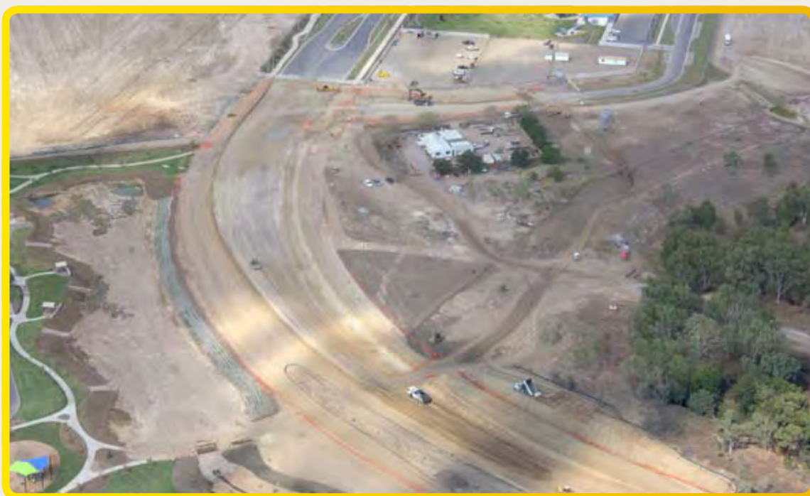
Construction crews have started work on a vital new road for the Northern Beaches.
