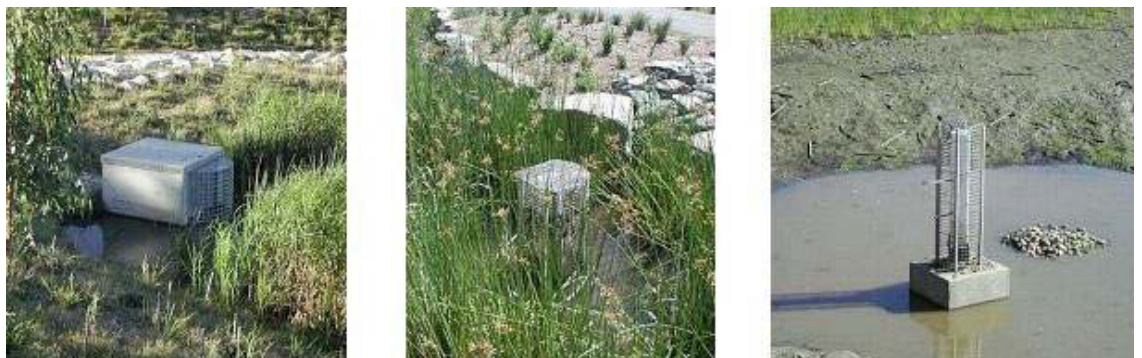
Plate 6-5: Example Outlet Riser Assemblies with Debris Guards
