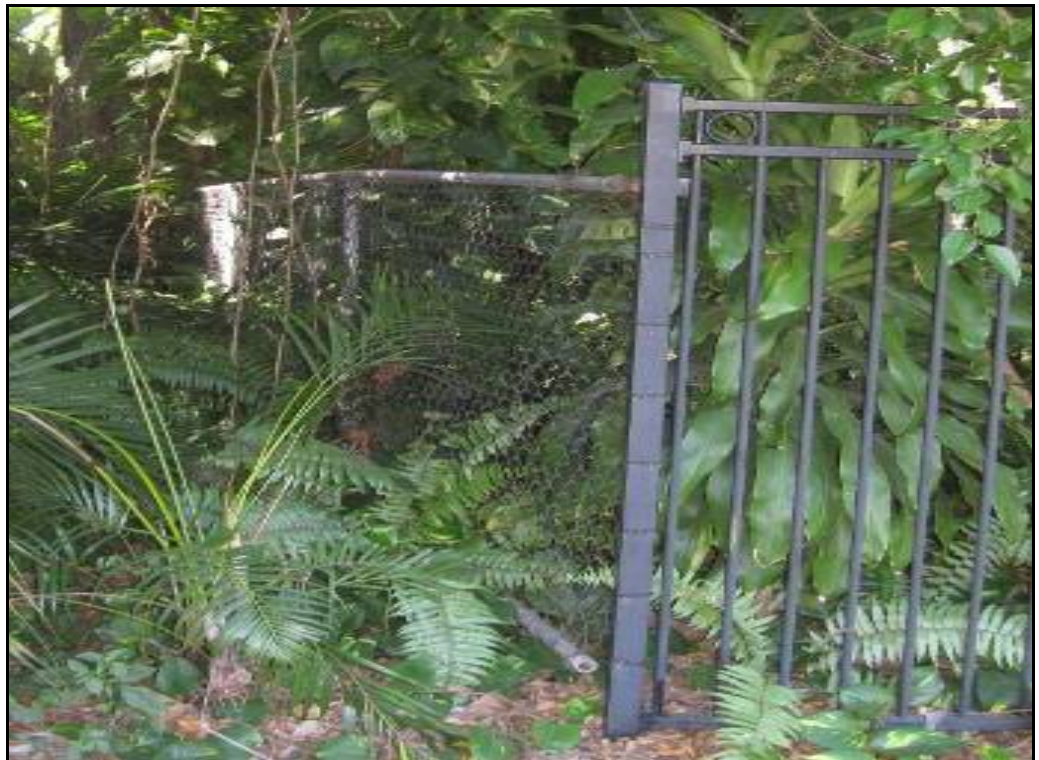
Figure 3.40 Junction between older chain mesh fence and more recent replacement - tubular steel fence panels (ERM 2010)
