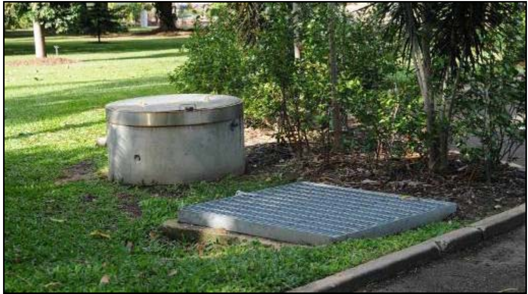
Figure 3.50 Well covered by grate and adjacent pump-housing (ERM 2010)
