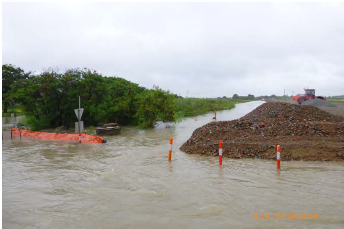
Photo 2 – Blakey St at Blakeys Crossing at 09.34 AM on 18 th Feb 2014 (the maximum flood level can be seen as a rough line on the embankment, several points along this line were surveyed post flood).
