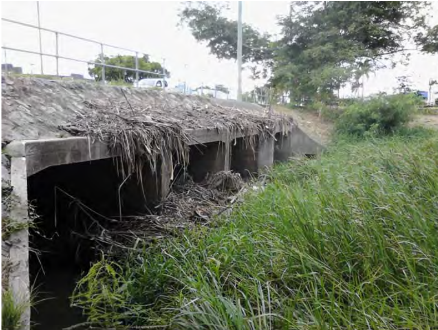
Photo 19 – Louisa Creek at Bayswater Road Culverts (upstream) showing debris following Feb 2014 event
