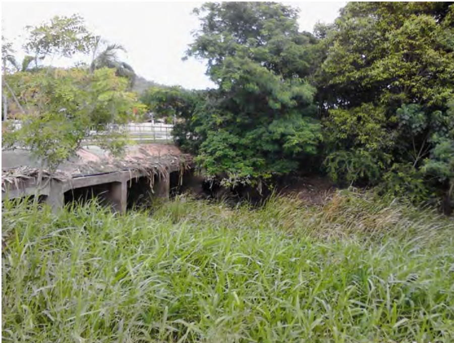
Photo 18 – Louisa Creek at Bayswater Road Culverts (downstream) showing debris following Feb 2014 event
