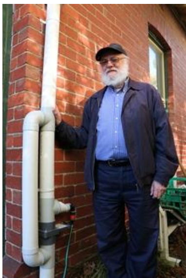
Figure 9-4 Downpipe Diverter - Meyer Rafael of St Kilda East says the condition of his soil has already improved after his downpipe diverter was installed. Source: City of Port Phillip.
