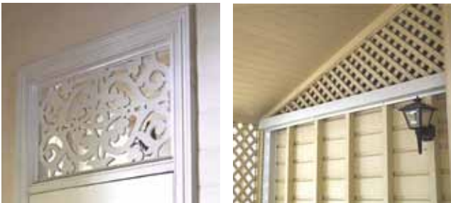
Figure 6 Internal vents and other openings can allow ventilation through the house when walls interfere with natural breeze flow (Photo: Kelly Goodbun).
