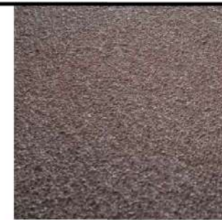
RND-01 PAINTED RENDER FINISH TO UPPER LEVEL BALCONIES AND FACADE TO BOTH BUILDINGS
