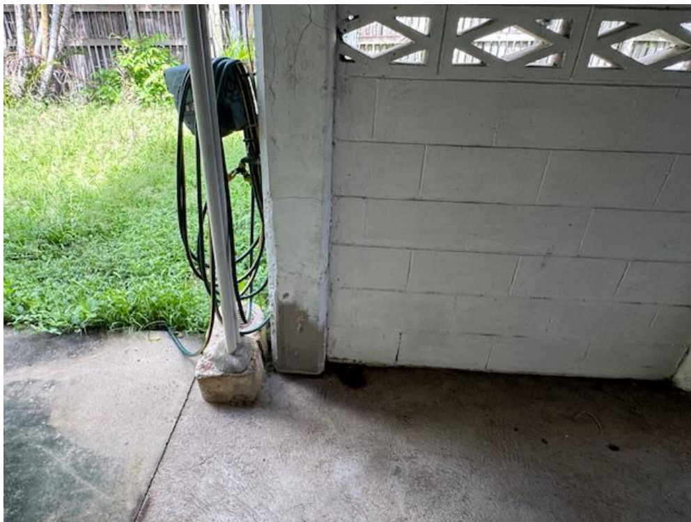
Figure 6 Evidence of concrete cancer
