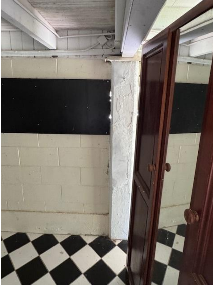
Figure 9 Evidence of concrete cancer
