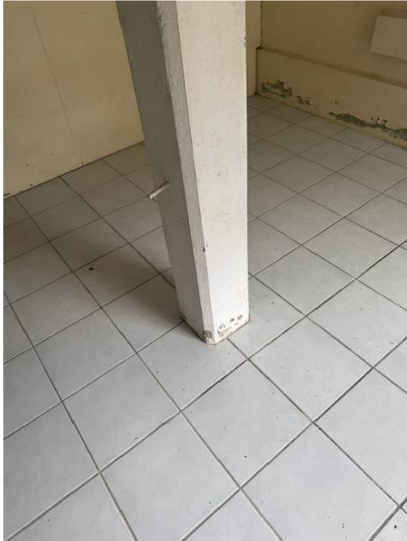
Figure 10 Missing Bracing & Bolt Protrusion
