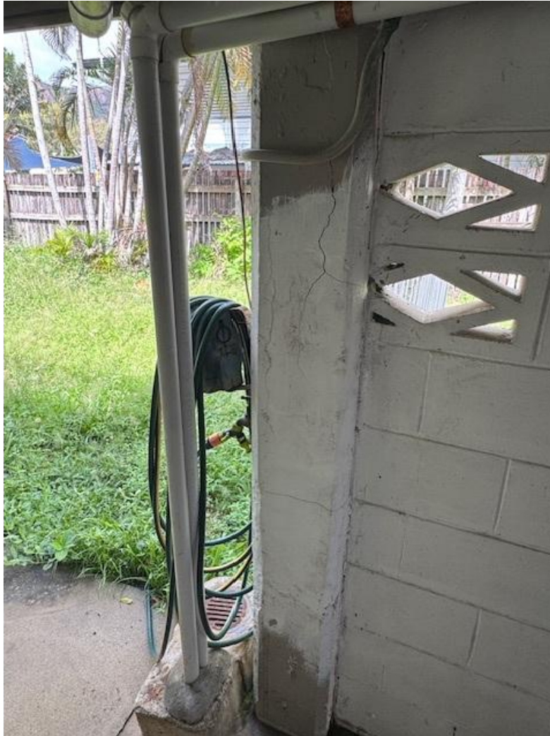
Figure 7 Evidence of concrete cancer
