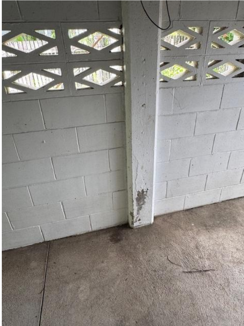
Figure 8 Evidence of concrete cancer
