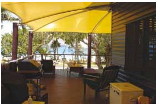
Figure 6 An example of where insulation would greatly improve the usability of an outdoor area. This low, uninsulated sail roof will radiate heat onto the deck area below. (Photo: ecoSAVVY).
