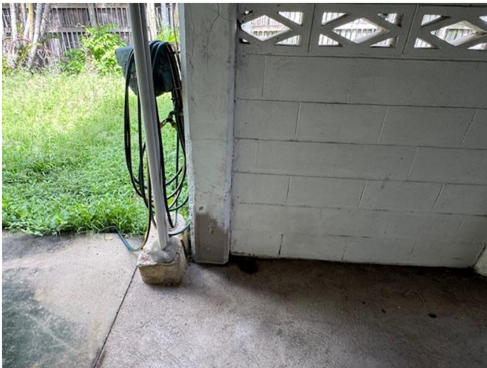
Figure 6 Evidence of concrete cancer
