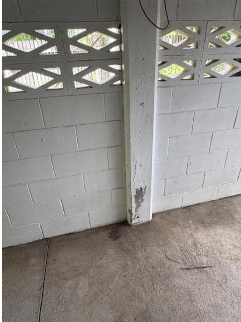
Figure 8 Evidence of concrete cancer
