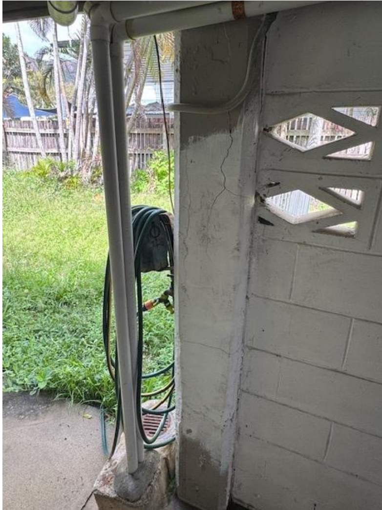
Figure 7 Evidence of concrete cancer
